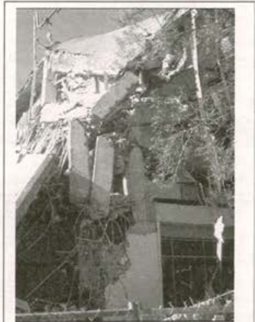
Figure 4 – Joint failures – Northridge earthquake
